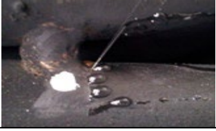
Failed weld or failed material covered under warranty
