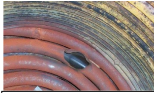
Pipe rupture due to freezing or obstruction
