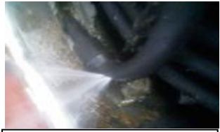
Blow out from pipe weakened by freezing
