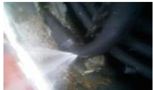
Blow out from pipe weakened by freezing
