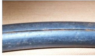
Failed pipe seam covered under warranty
