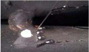
Failed weld or failed material covered under warranty
