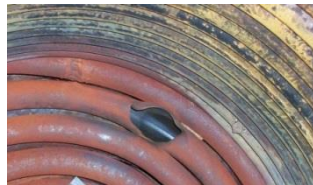
Pipe rupture due to freezing or obstruction
